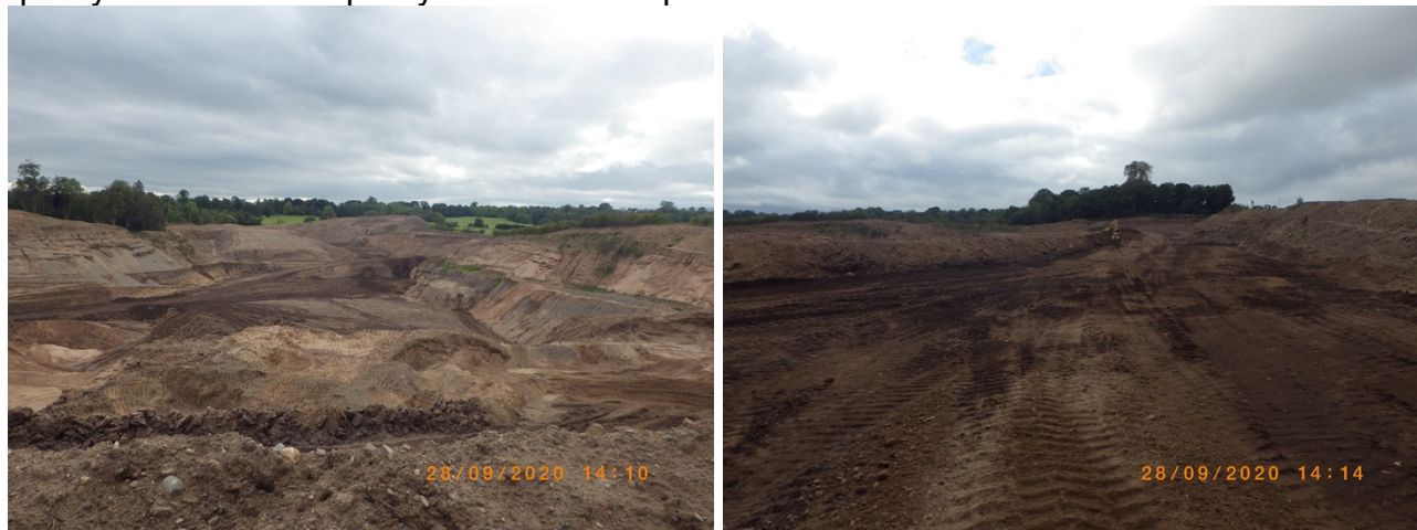
Excavated area where Inertia site was (photo 1 looking south, photo 2 looking west)
