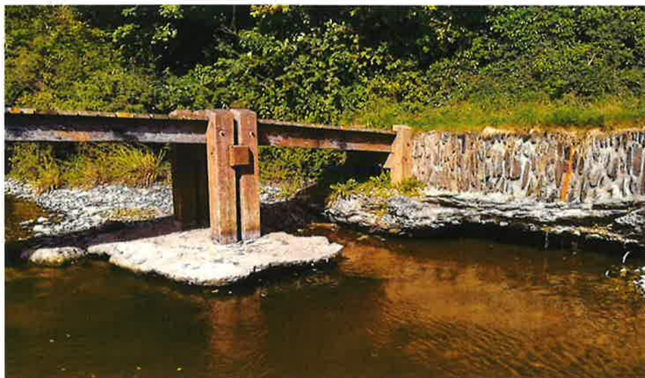
Photo 1 – Scour of bridge and pier foundation (Summer 2019)
