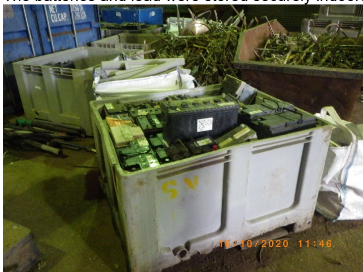
Indoors battery storage
