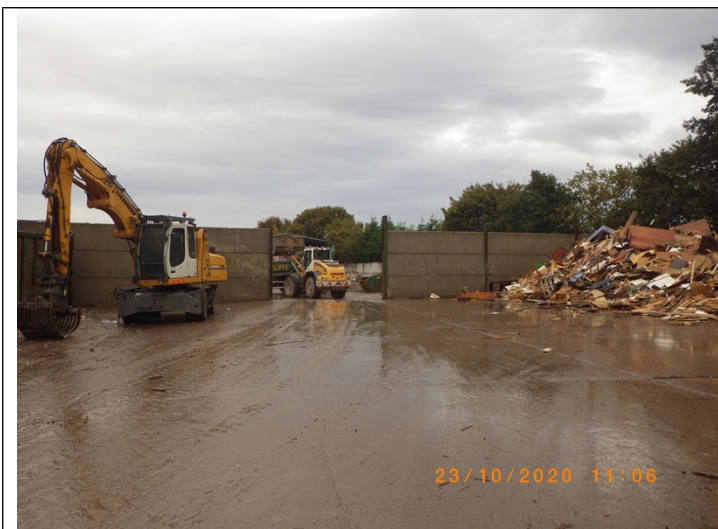
Part of wall missing adjacent to wood pile
