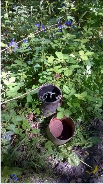
GW6 with missing lock.
