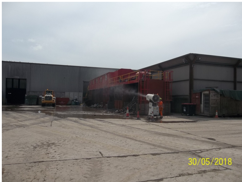
Photo 1: New processing unit located in the yard, with dust suppression equipment in operation.
