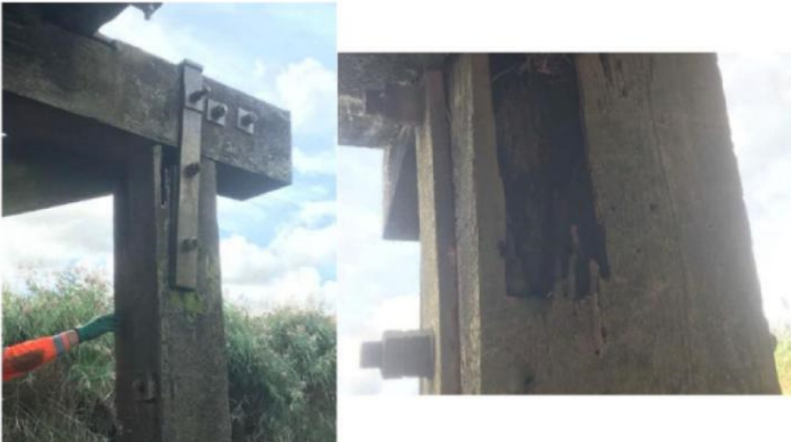
Figure B.11 – Trestle 3 Pile 6. Decay to bearing area at crosshead, loss of contact area.
