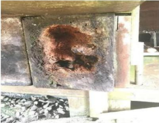
Figure B.4 - Heavily decayed main beam outer corbel (Main Beam 2). Requires replacement in the next 6 months.
