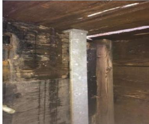
Figure B.5 – Edge beam loss of section and heart rot over bearing interface with upper corbel.
