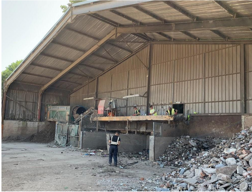
Plate 5-3 Trommel and Picking Line in Building
