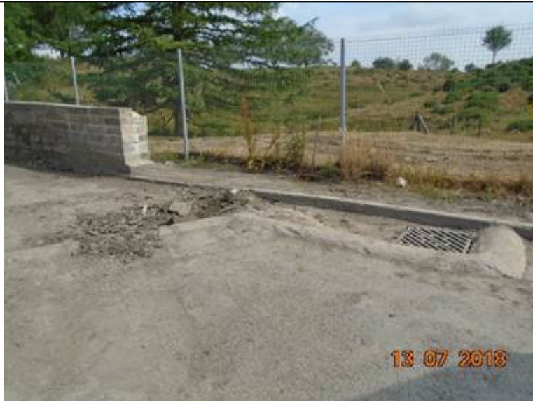
Image 2 – Clear drain, though small accumulation of mud/silt which may hinder drainage in wet conditions.
