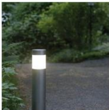
Plate 1: Example of low level lighting provided by bollards
