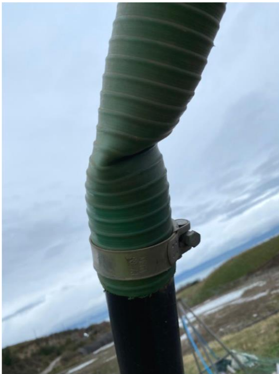
Photo 2 – D318 kinked pipework
