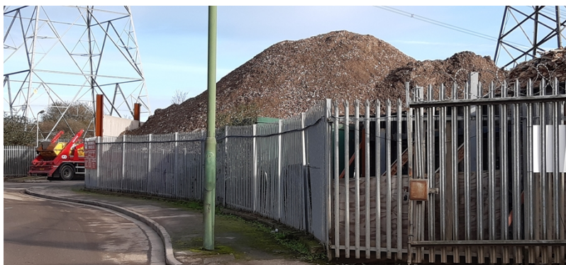
Photo 6 - Stockpile of waste within 1 metre proximity of site boundary
