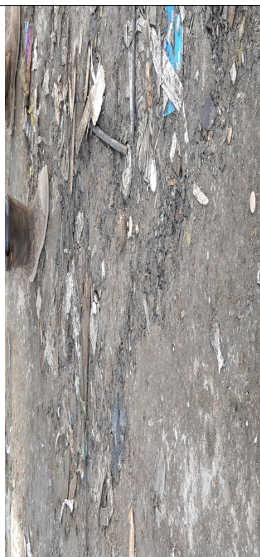
Photo 4 - Concrete flooring at GD Environmental requiring attention
