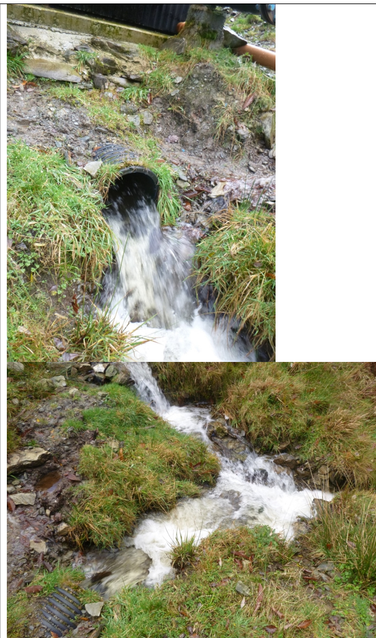
Figure 3 & 4: Discharge outlet pipe
