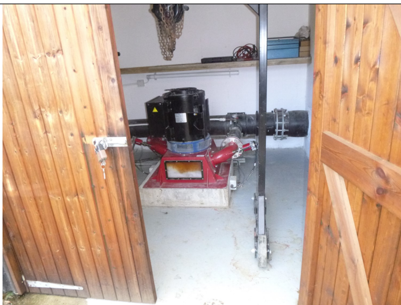
Figure 2: View into the turbine house
