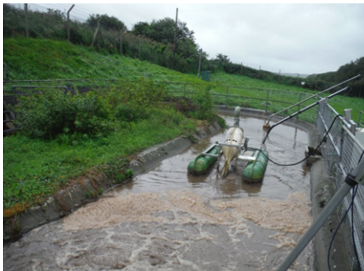
Photo 1: Raft aerator within the activated sludge ditch
