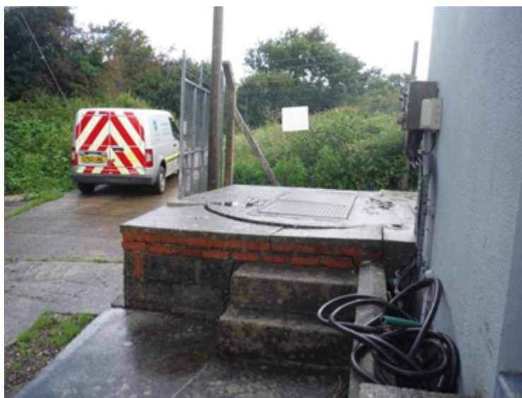
Photo 2: Cracked outer wall on the inlet chamber. Cracks start at top of steps and go down the side of the chamber to at least ground level.
