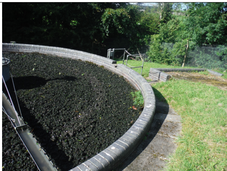
Photo 2: Missing brickwork can be seen on the right of the filter bed wall.
