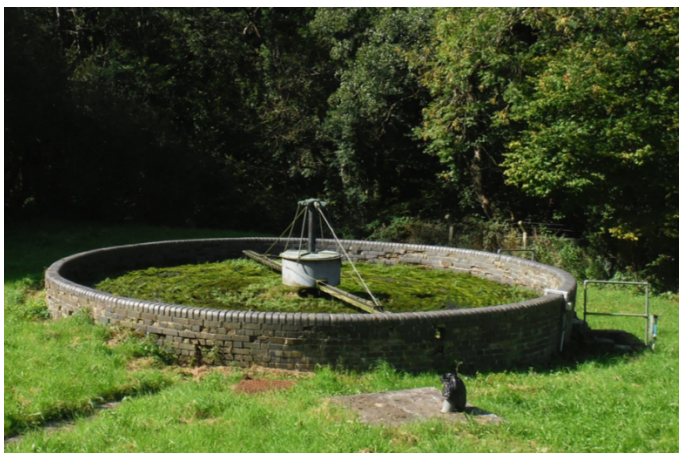
Photo 1: Crumbling and cracked brickwork on filter bed. Also, there was a thick growth of moss on the filter media.
