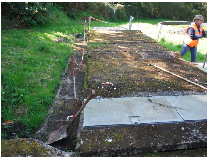
Photo 2: Brittle and weathered looking concrete lid of the septic tank. The structure has been cordoned
