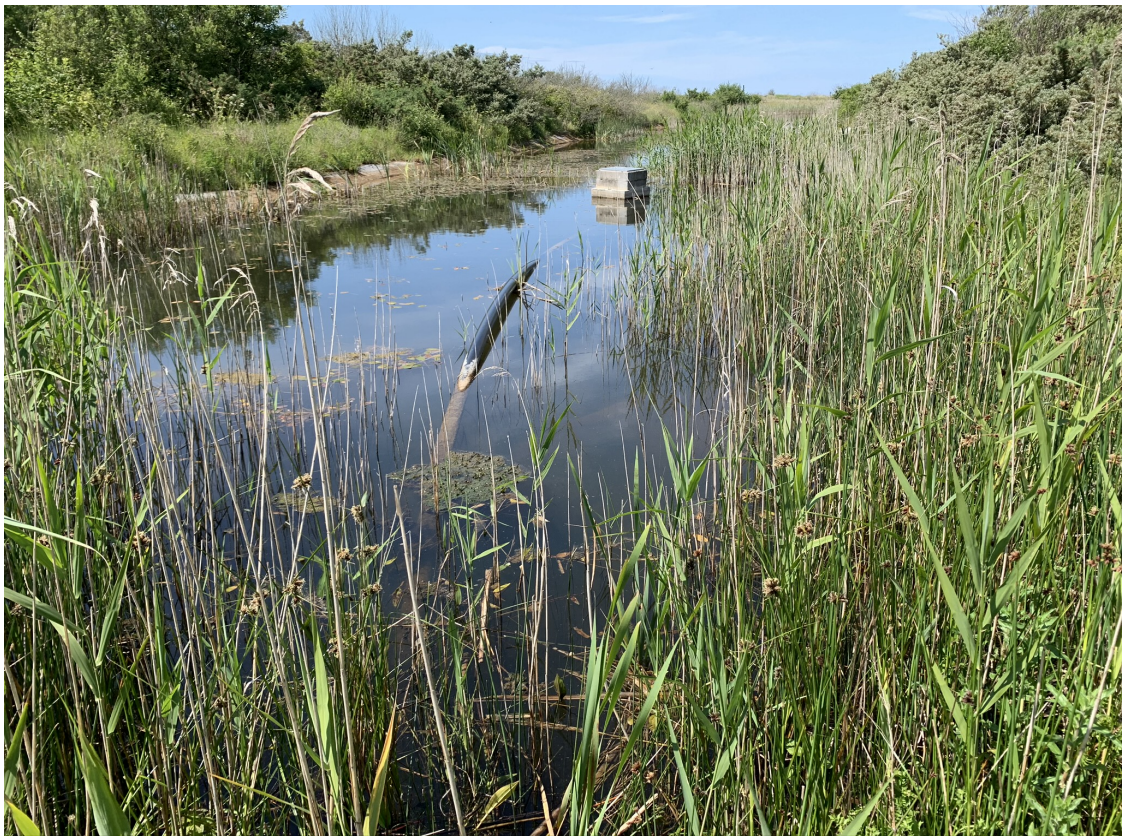
Plate 4-3 Intake chamber in Pond 3
