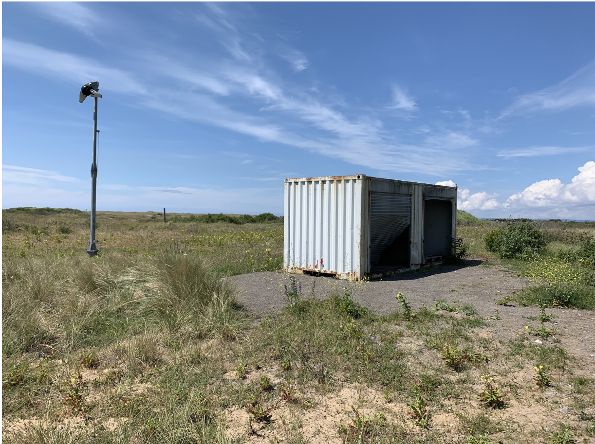
Plate 4-6 Damaged wind turbine and control room
