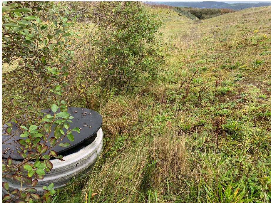
Plate 4-5 Pipework chamber in valley between MCL and Biocell
