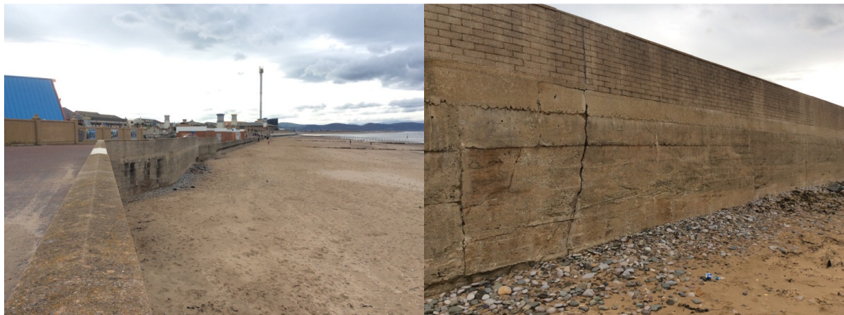
Figure 2-5 Cracking in defence fronting the SeaQuarium, Central Rhyl.
