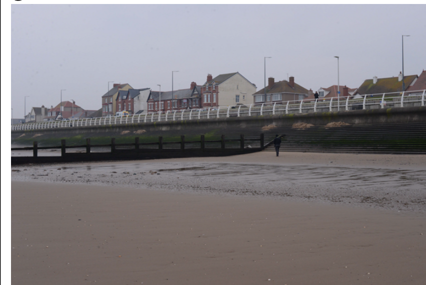
Existing stepped revetment not currently providing adequate flood protection.
