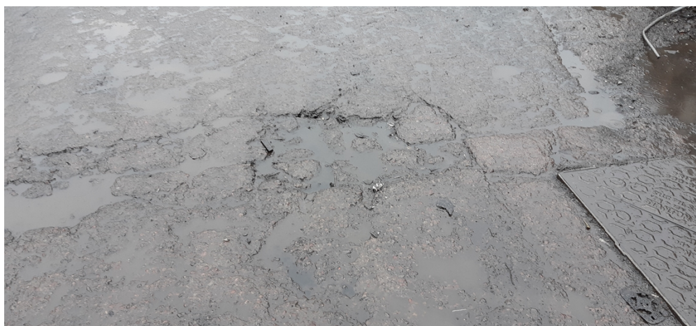
Photo 3 - Damaged flooring located on site
