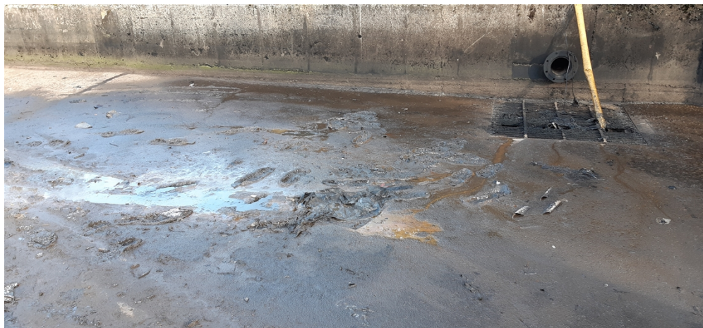
Photo 1 - Residual sludge containing traces of oil from recent flooding event
