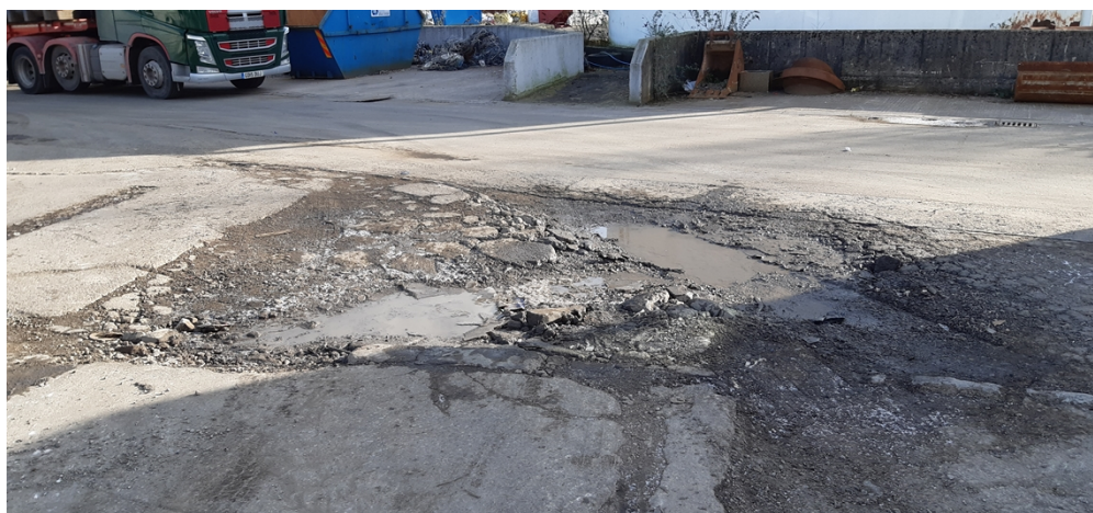
Photo 2 - Damaged flooring located on site
