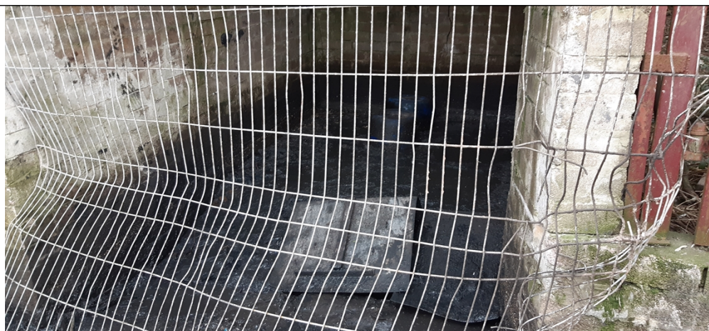
Photo 2 - On site interceptor drainage system
