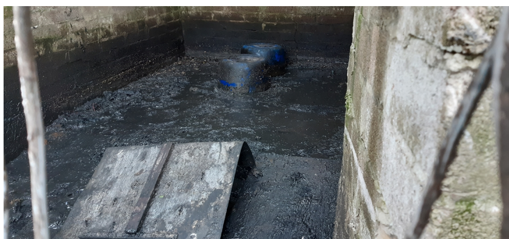
Photo 3 - On site interceptor drainage system
