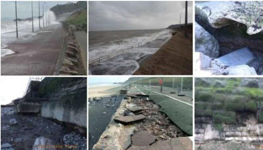
Figure 1.2: Examples of Old Colwyn Promenade Storm Damage
