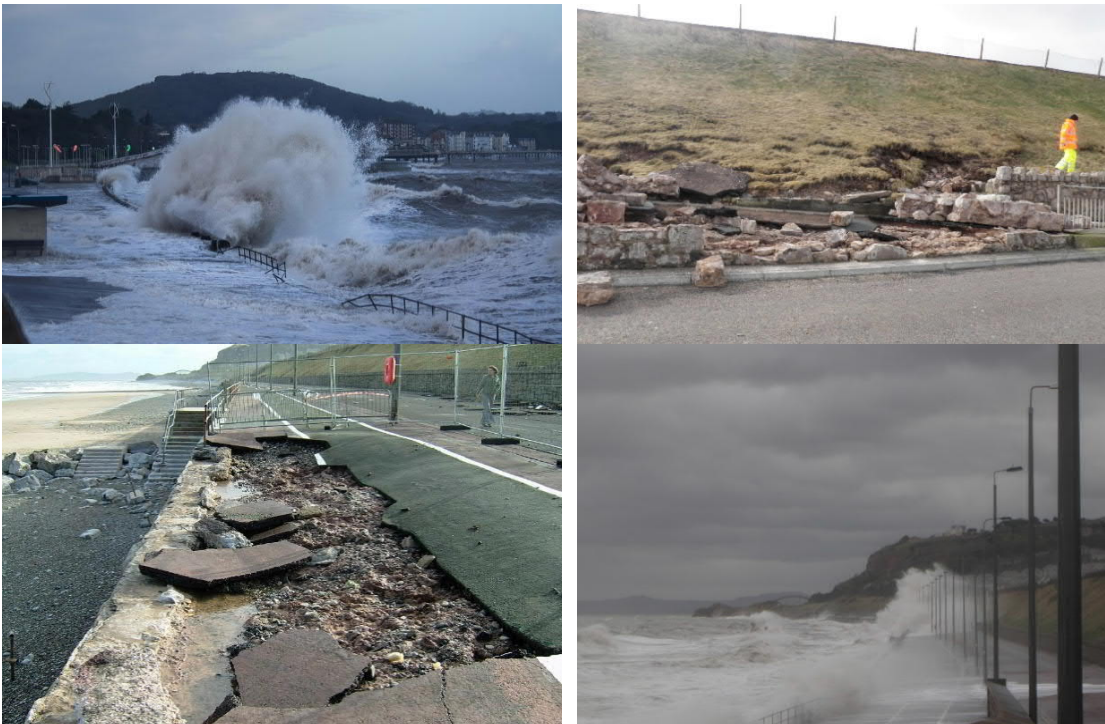
Figure 1.1: Examples of Coastal Overtopping and Damage at Old Colwyn
