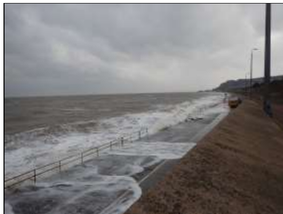
Damage to railings
