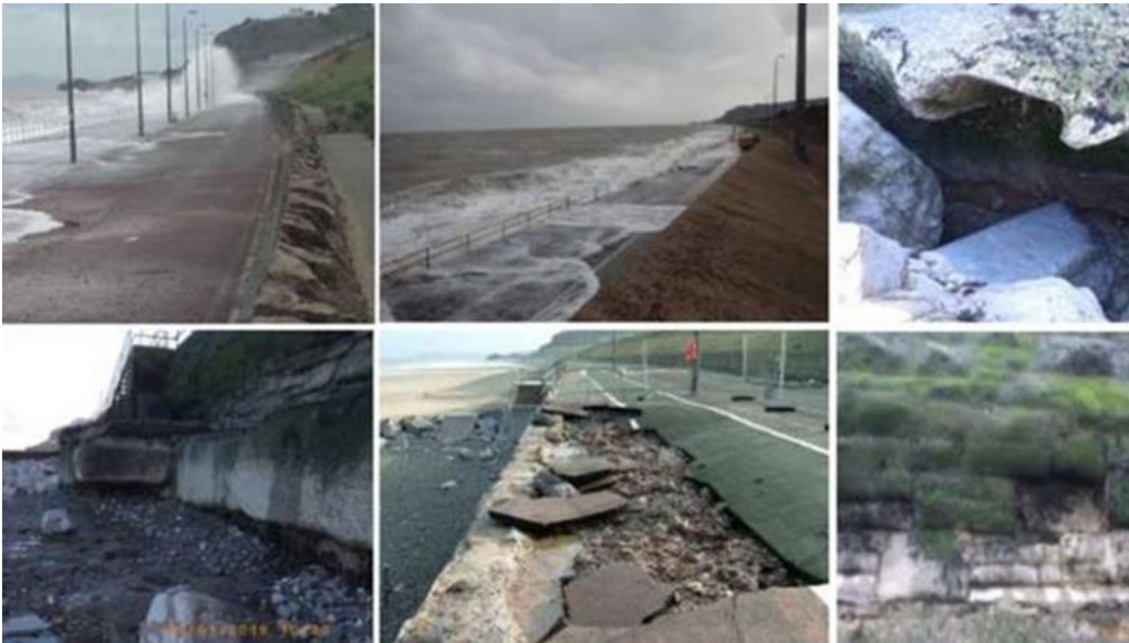
Figure 3-3: Old Colwyn's sea defence damaged during a storm
