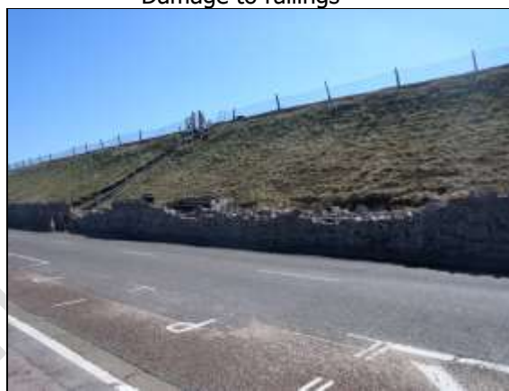
Damage to NR boundary wall and embankment
