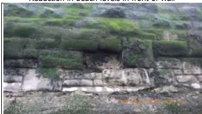
Loss of Blocks to Sea Wall
