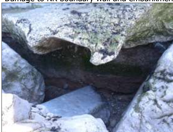
Sea Wall Undermining
