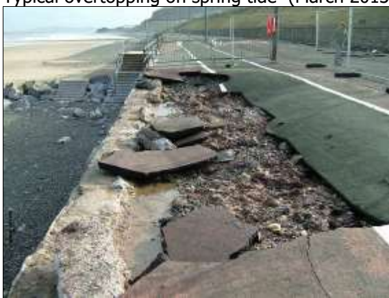
Damage to promenade surfacing
