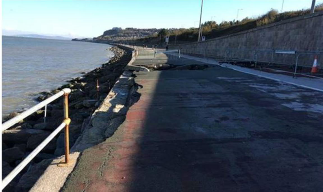
Figure 2.2: Example of Old Colwyn Promenade Storm Damage
