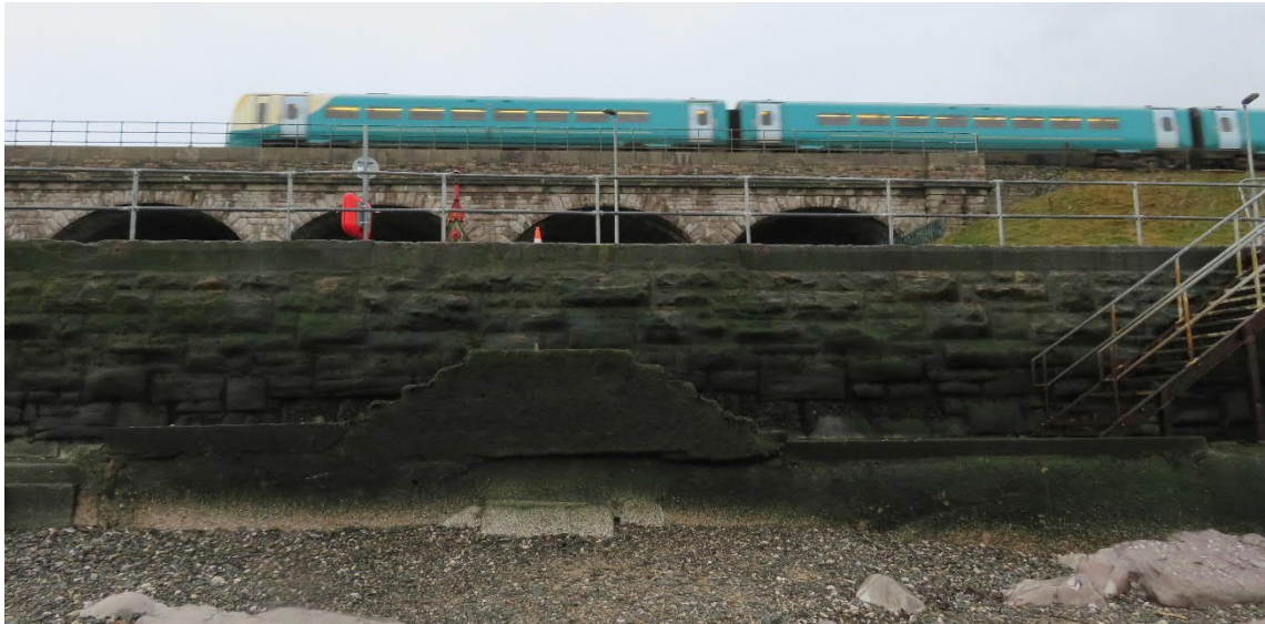
Photo 1.9: Looking South at Splashpoint Sea Wall with NWC Railway Bridge to Rear
