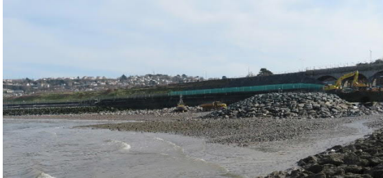
Photo 1.8: Looking South-East Across the Transition between the Existing Splashpoint Revetment (Area 2) and the Area to the East of the Scheme
