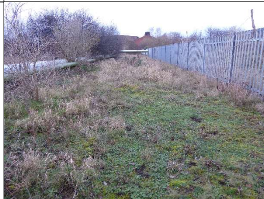
Photo. 38. Rabbit grazing and diggings around above ground steam pipe
