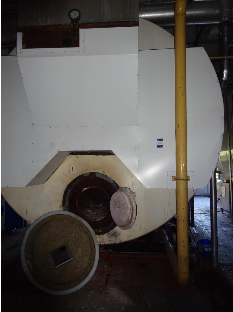
Arla, Llaandyrnog Final site inspection 16.04.2021 Photos 24 &25 – duty and standby boilers
