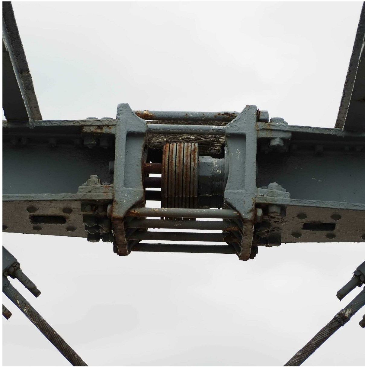
Typical In-situ condition For typical repair detail of element shown refer to drawings B072084-CUR-ZZ-ZZ-SK-D-27118/119
