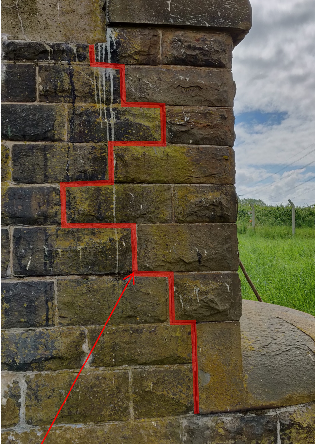
Cracked Masonry Example
