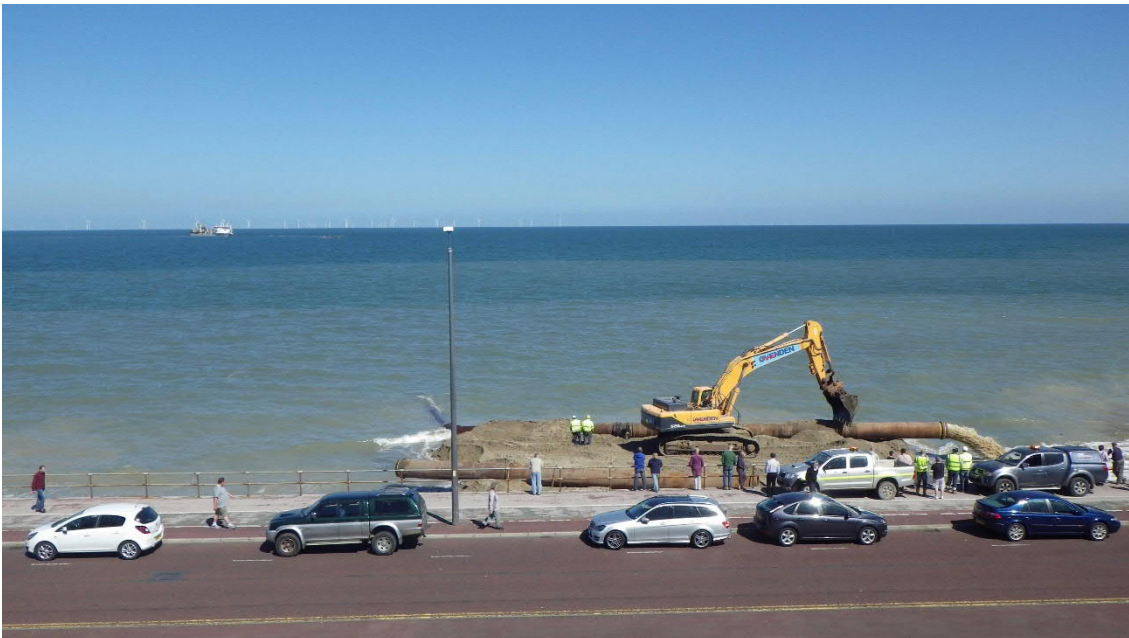
Photo 2.3: Beach recharge works during previous phase – view from shore of the sinker and shore pipelines with the TSHD and floating line in the distance
