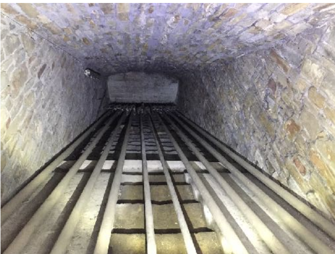
View of chamber that holds cables
