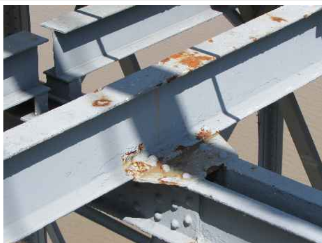
Main Boom Primary Steelwork Corrosion at interface between steel members.
