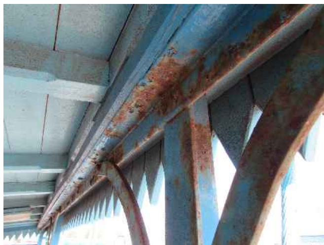
Gondola Topside Corrosion to framework members.
