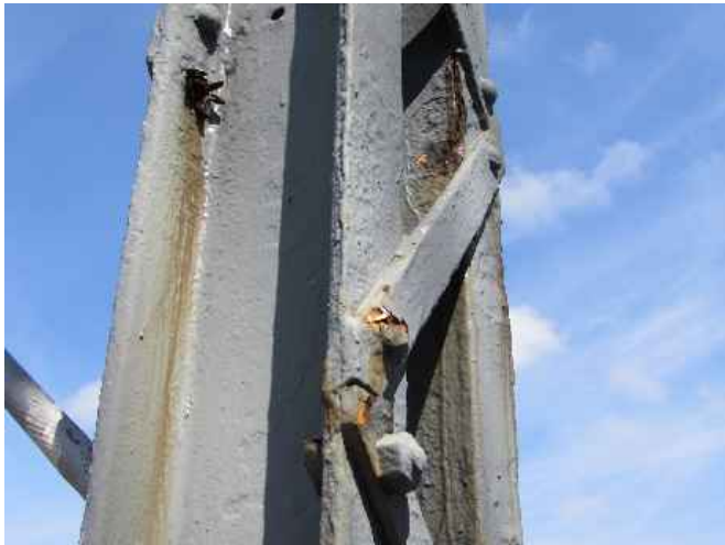
Main Boom Vertical Steelwork Corrosion and breakdown.
