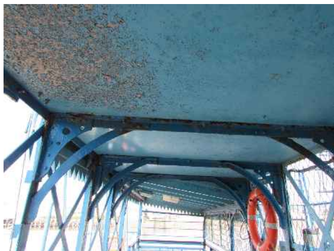
Gondola Topside Covered seating, deck plate showing coating delamination and flaking.
