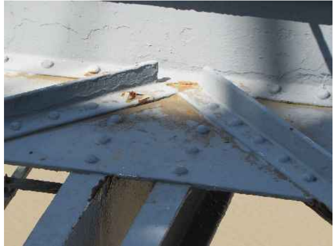
Main Boom Traveller Steelwork Overview of corrosion.
