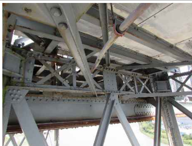
West Pylon Overview of underside, corrosion on edges, joints and fixings.
