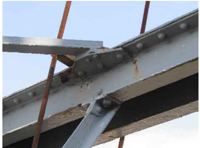
Main Boom Vertical Steelwork
