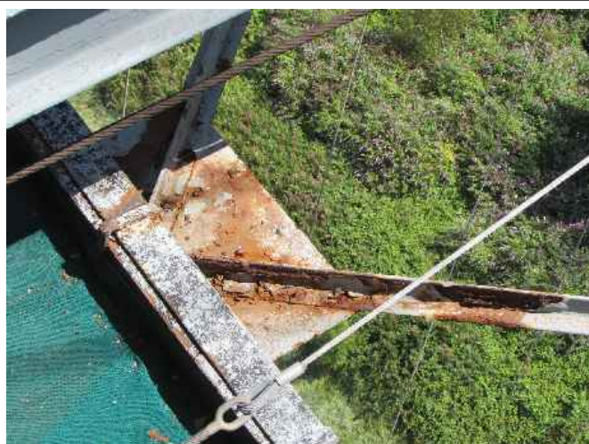
Main Boom Primary Steelwork Heavy Corrosion on main boom steelwork.
