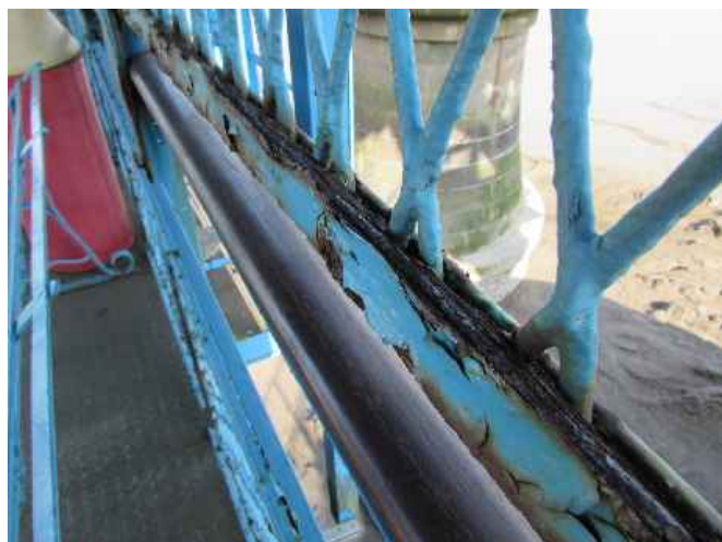
Gondola Topside Heavy corrosion and breakdown.
