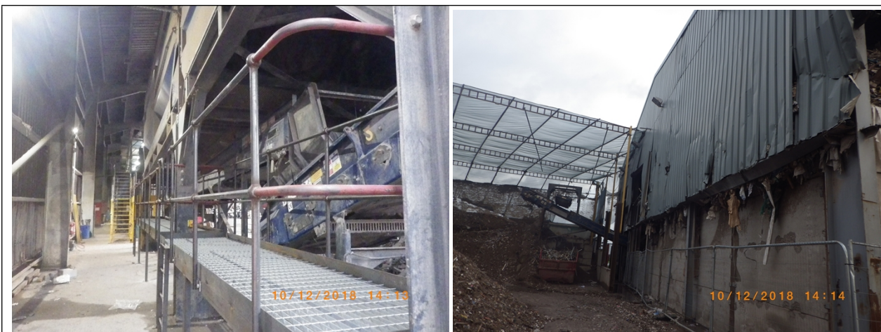
Conveyor line railings and panelling
