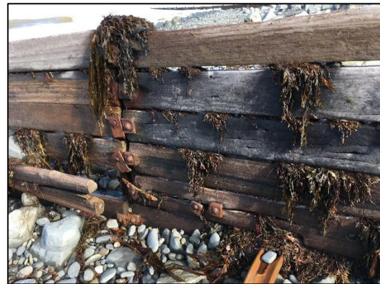
Figure 1-8 Weathered Groyne along South Beach
