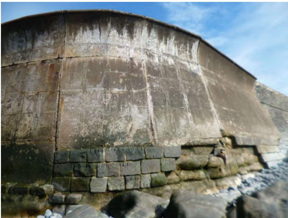
Insert 6-9 Detail of seaward end of the South Pier (Asset 9) showing rebuilding and poor condition
