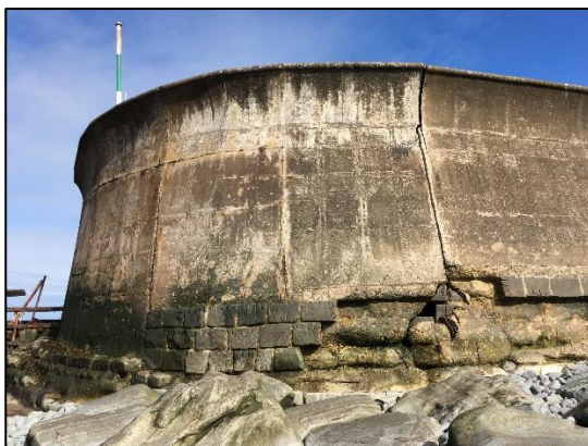
Figure 1-5 Dilapidated South Pier
