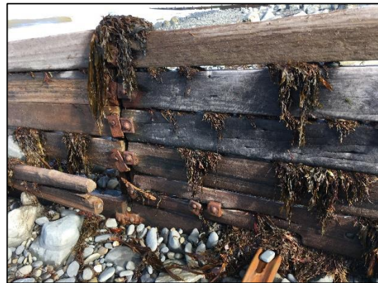
Figure 1-8 Weathered Groyne along South Beach
