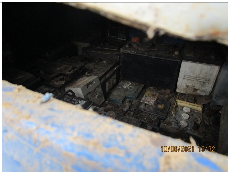
Figure 4. Batteries stored in acid resistant containers with a lid.
