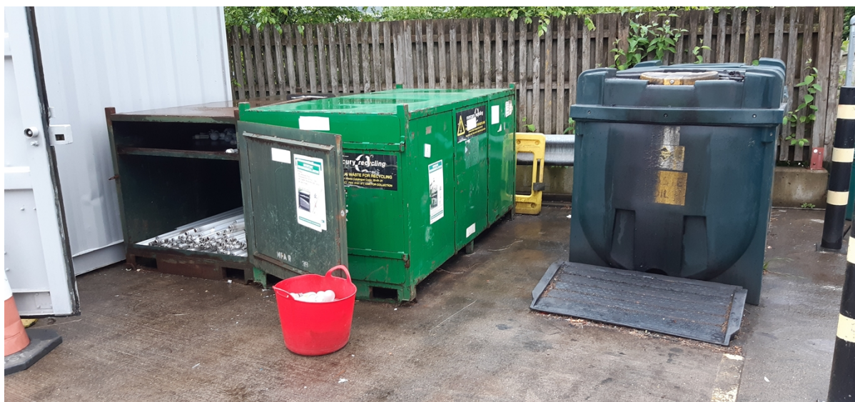
Photo 4 - Oil waste storage within interceptor drainage system area
