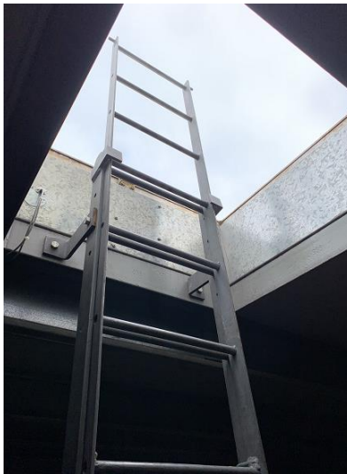
Image 9 showing extended access ladder
