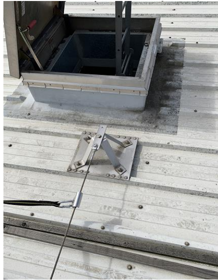
Image 10 showing roof access hatch and start of the Safeline fall prevention system.
