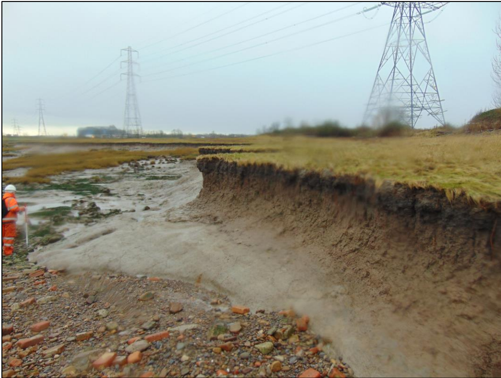
Plate 13: Eroding land surface on the eastern bank of the River Rhyrnney, view to southwest.
