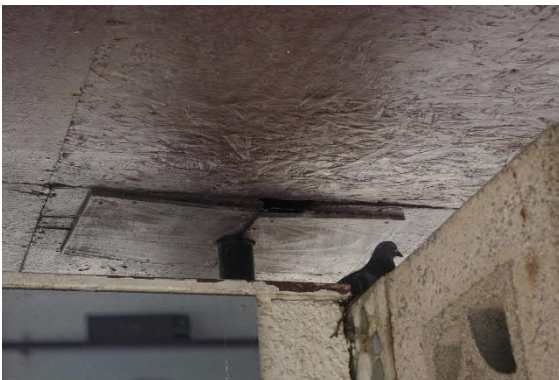
Figure A.15: Gap in plywood and nesting feral pigeon (B7)
