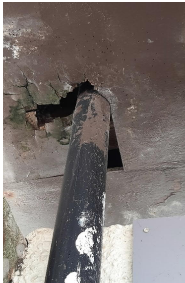
Figure A.8: Cavity surrounding drain pipe (B4)
