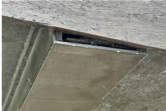
Figure A.10: Cavity within soffit box on south-east corner (B5) Note: during the period of rain, water was pouring out of this cavity
