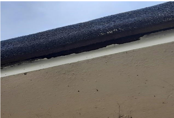
Figure A.3: South facing gap in roof (B2)
