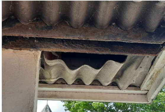
Figure A.6: Dropped roof void on south-west side (B3)
