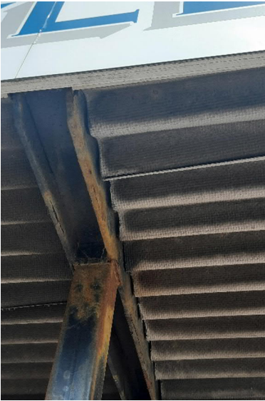
Figure A.5: Gap on north-east side (B3)
