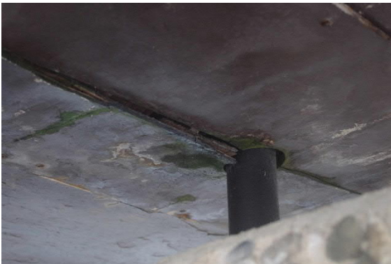
Figure A.11: Cavity around drain pipe with leaky roof (B5)
