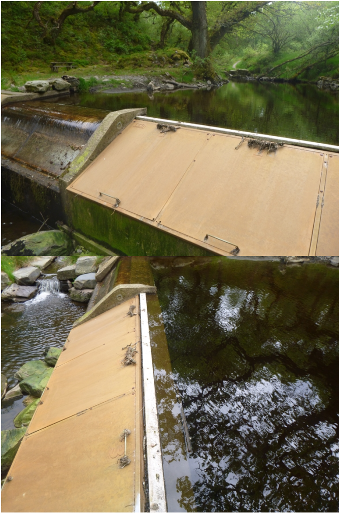
Photograph 3: Increased height of residual flow section Photograph 4: Increased height of residual flow section
