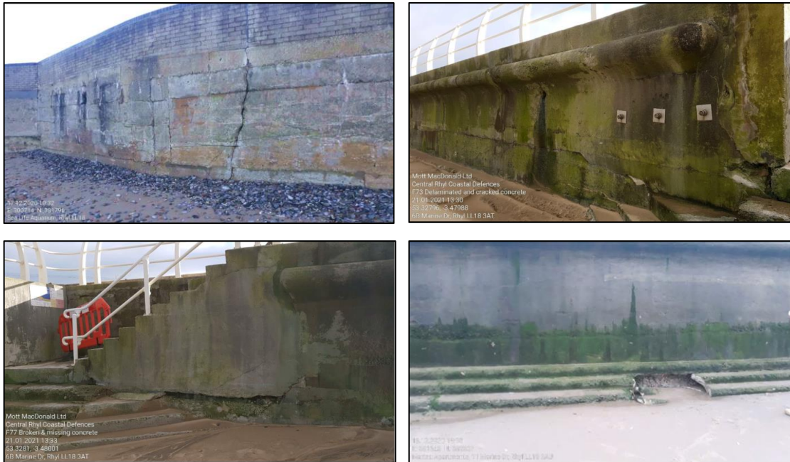
Figure 1.2: Deteriorating defence condition along the Rhyl frontage
