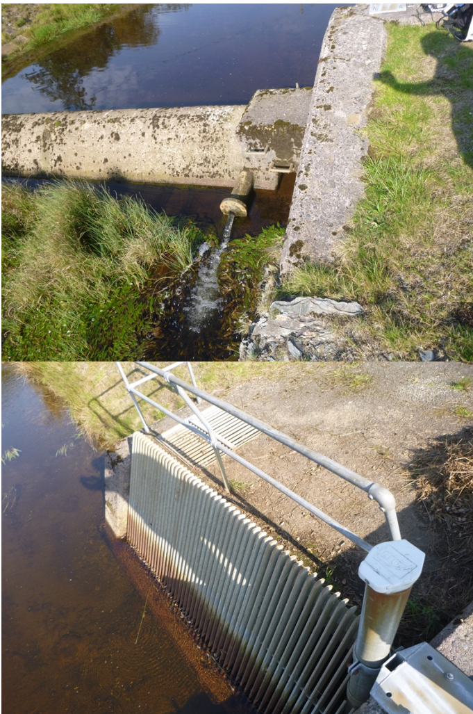
Figures 3 & 4: Orifice plate and abstraction screen at Afon Llywernog
