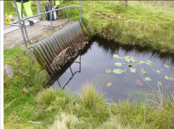
Figure 13 & 14: Outfall and screen at Llyn Bygeilyn
