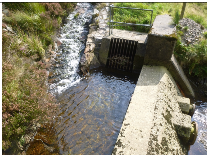
Figure 11 & 12: Intake and orifice plates at Hengwm
