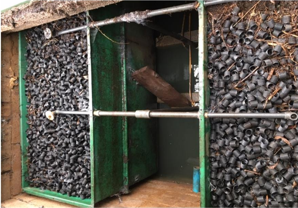
Photo 3: Trickling filters closest to inlet in Secondary Treatment System (covers removed)
