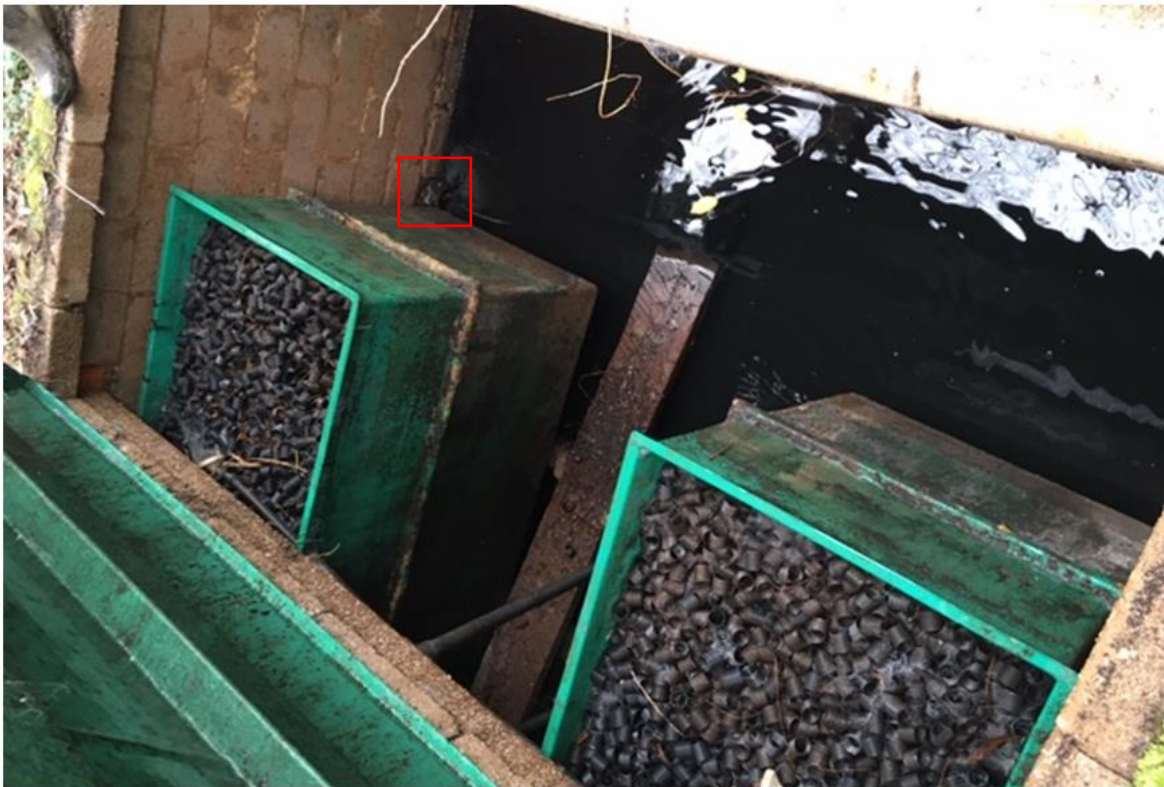
Photo 4: Trickling filters closest to outlet (in red) leading to discharge point in Secondary Treatment System (covers removed)
