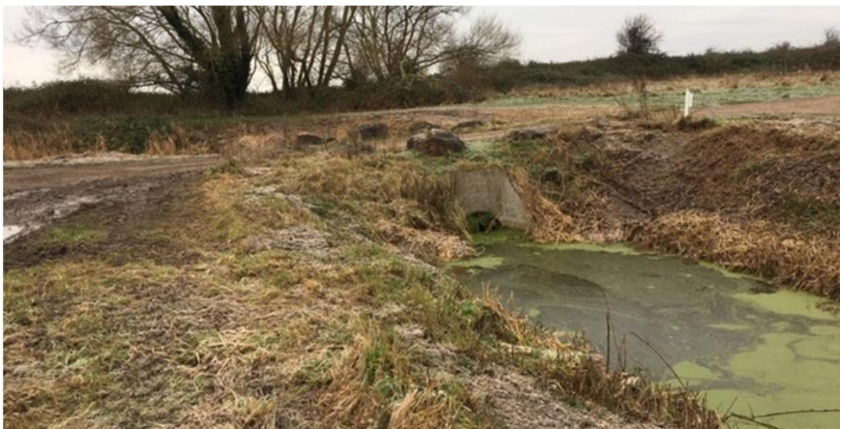
Photo 6: Reen connected to discharge reen. Reen smelt of sewage.
