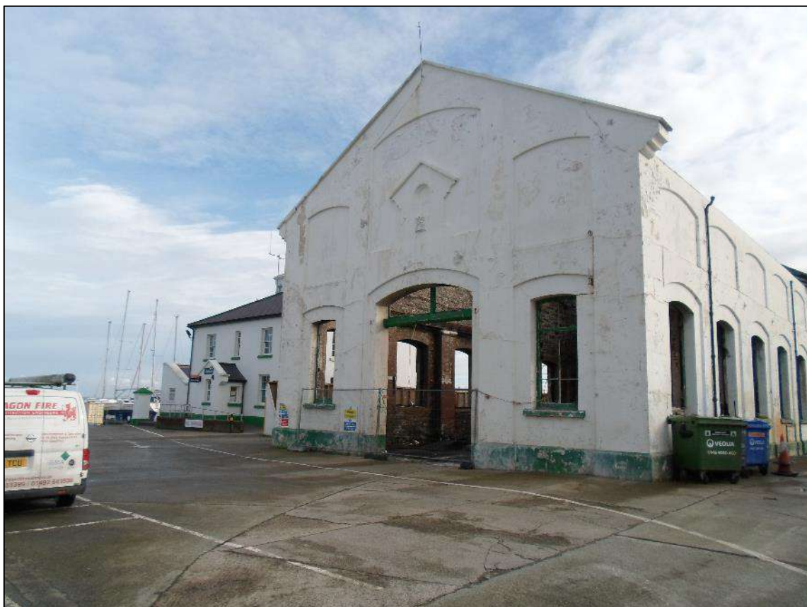
Plate 18. Fire damaged Trinity Yard Large Workshop (LB 14731) looking north-east
