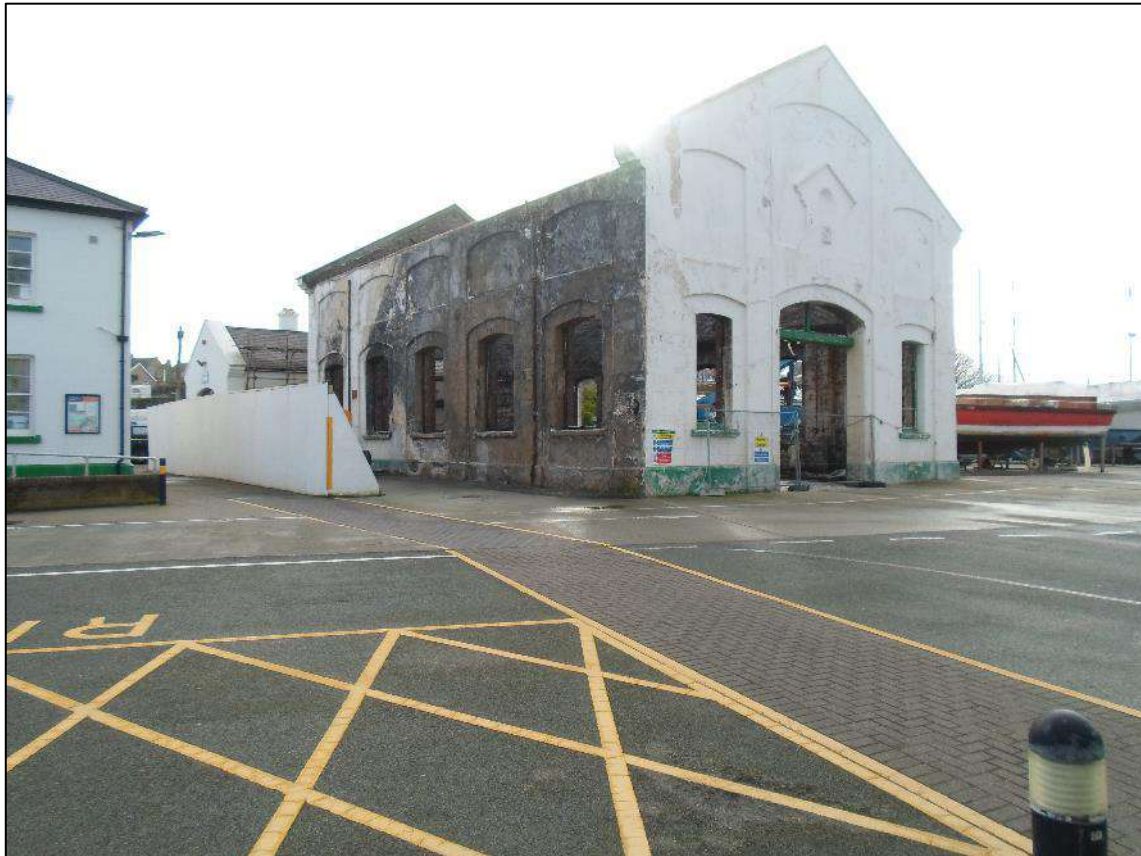
Plate 17. Fire damaged Trinity Yard Large Workshop (LB 14731) looking south-east
