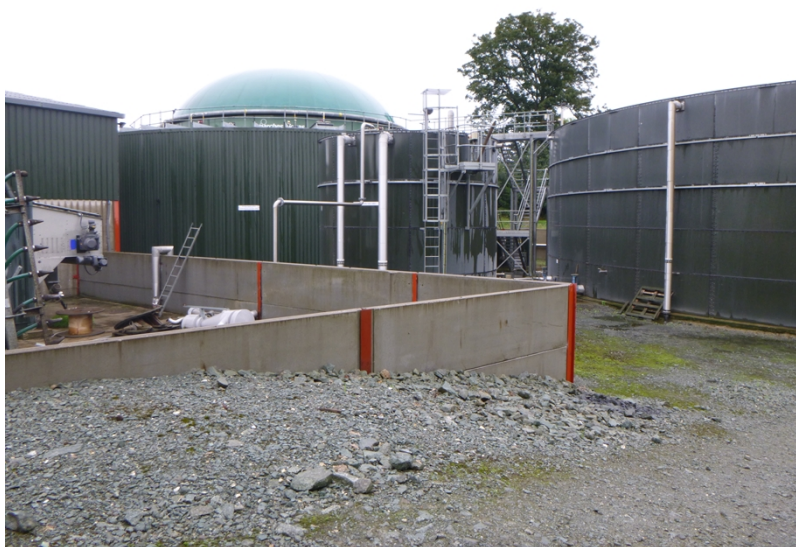
Image 2: Bunded digester (left) and slurry store (right)
