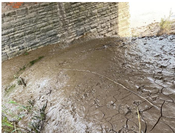
Figure 15: Animal prints/tracks beneath second arch (Newport side)
