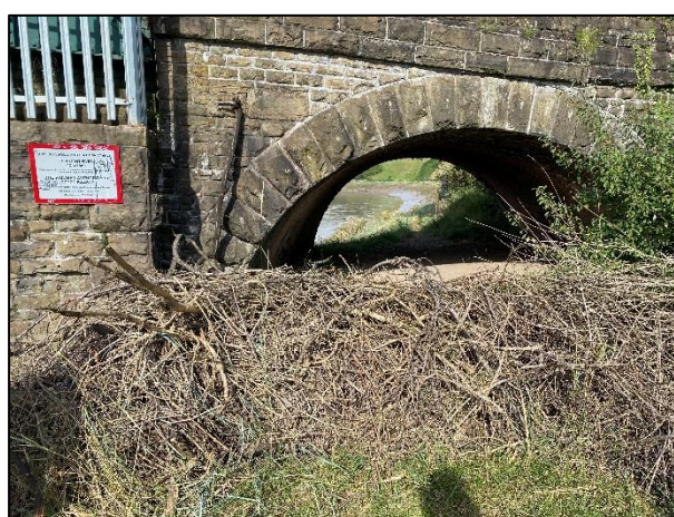
Figure 14: North bank arch and debris
